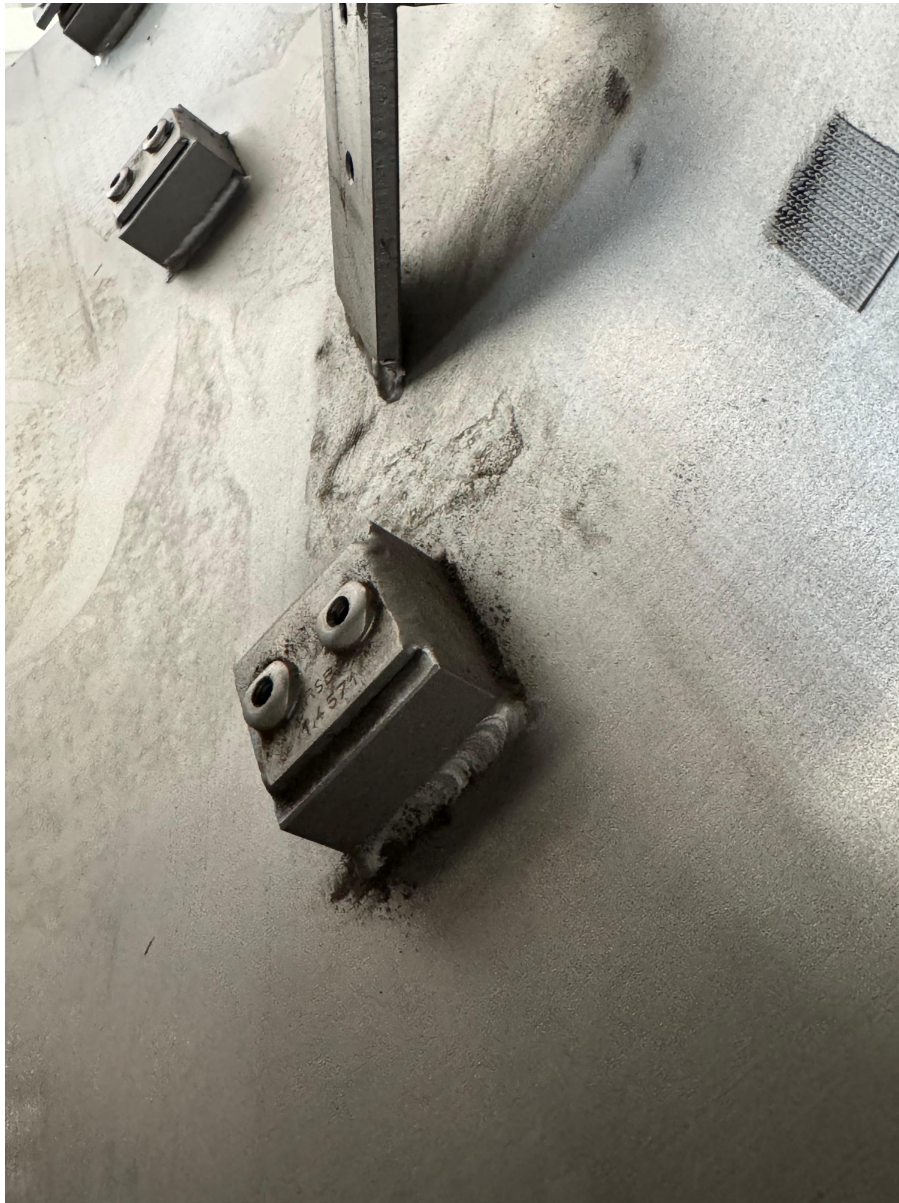
Figure B.2 A close-up of the attachment point depicting some contamination from previous shroud system as well.
